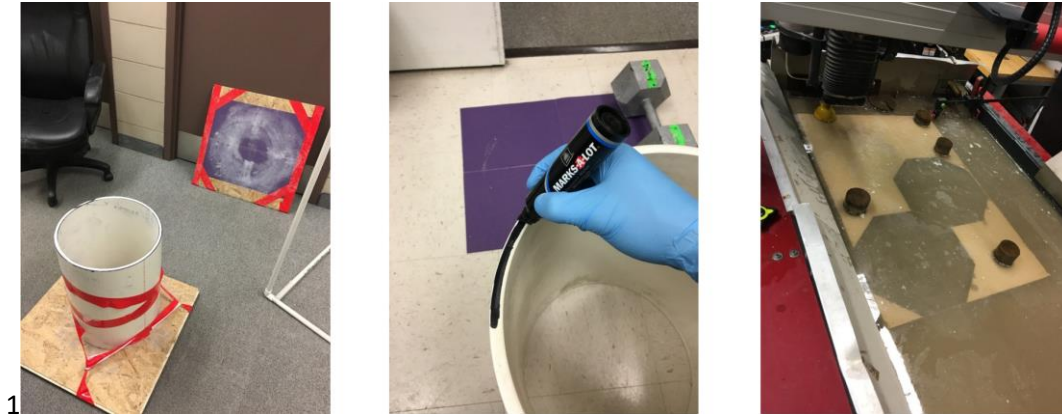
Fig. 2: Sanding the PVC pipe and cutting out Lexan endplates with a waterjet cutter, following Brooks' design [Ref. 1].
