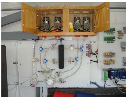
Figure 2. Instrumentation inside of a Mobile Air Emissions Monitoring Unit.
