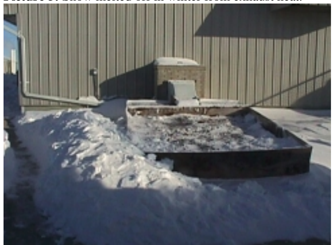
Picture 5: Snow melted off in winter from exhaust heat.
