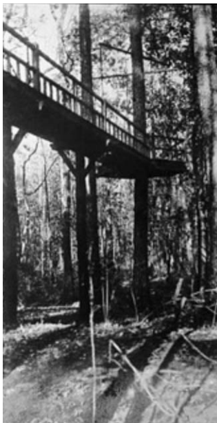
Bridge or walkway structure, as it extended at grade into the woods.
