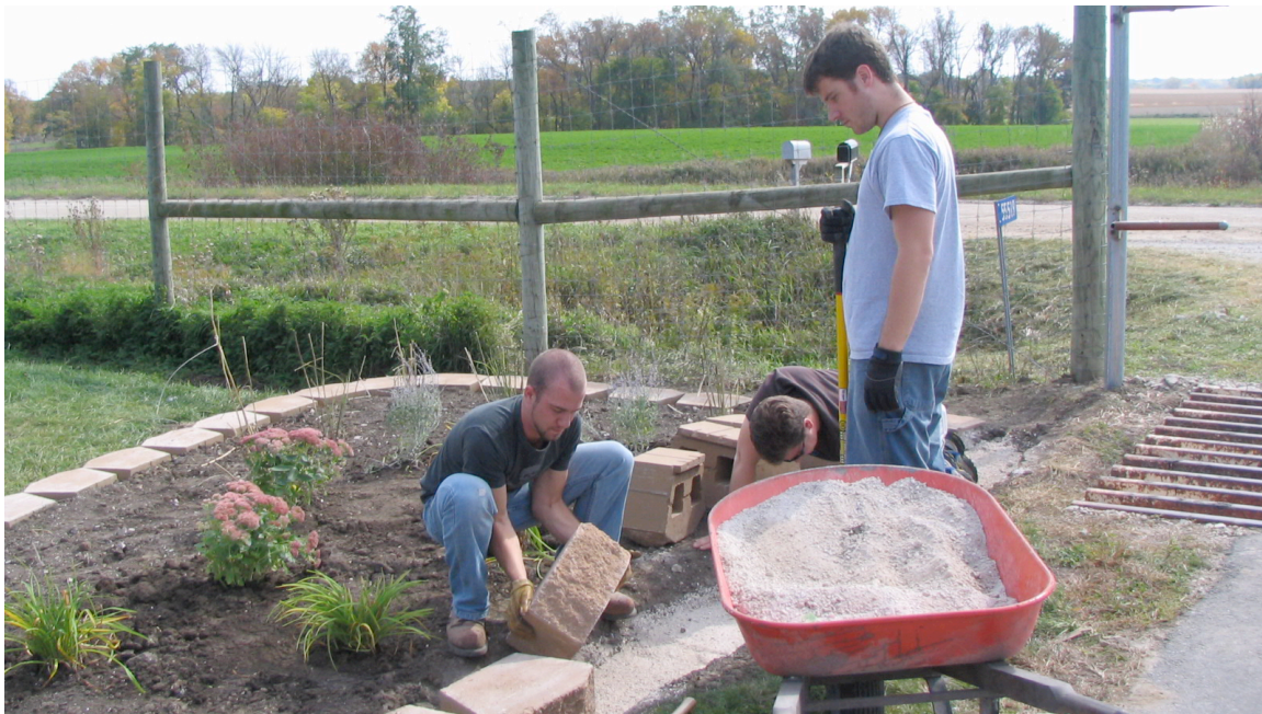
Figure 1. HORT 444 Monday lab section students installing the final blocks of the retaining wall.
