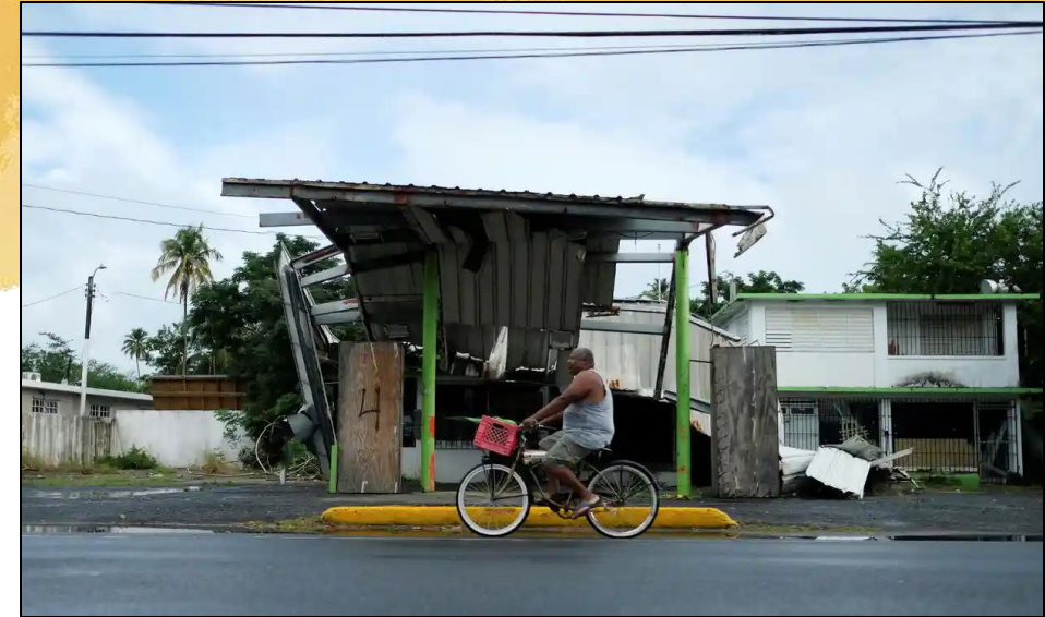
Gas station damaged by Hurricane Maria
