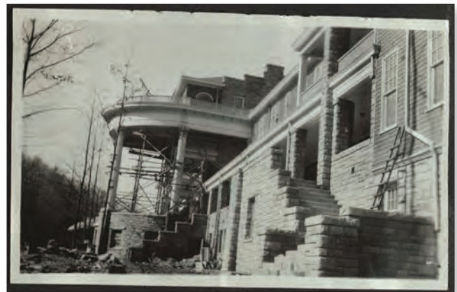
The front balcony and staircases to the hotel in Lynch, meant for visiting company executives. In this photograph, the front balcony is under construction, page 32. Courtesy of The Filson Historical Society.
