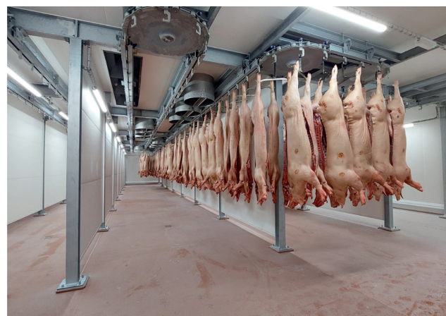
Figure 3. New installation of a contemporary quick chill tunnel for effective chilling of pork carcasses with minimal power use. Cooling relies on direct expansion ammonia and the cooling space has been diminished by a horizontal deck in the cooling tunnel. This will lower energy consumption by up to 30% and make cleaning and maintenance easier. An efficient quick chill tunnel should have a chill loss of 1.0% or less.
