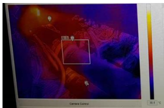
Figure 6 : abnormal monitoring using a thermal imaging (ex)
