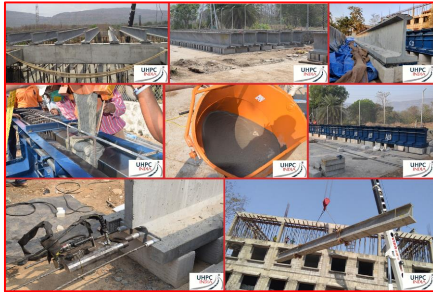
Figure 7 Pictures from site showing the different steps during UHPC beam casting, post-tensioning and erection (With permission from UHPC India Pvt. Ltd., Mumbai (India))
