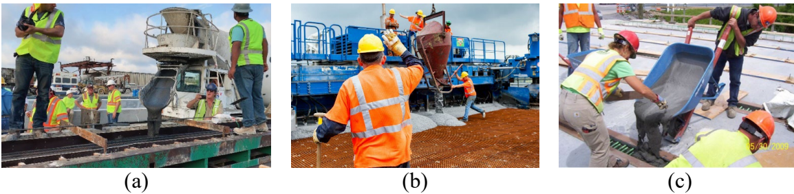
Figure 2 Different casting devices for large scale UHPC construction (a) inclined chute or half-pipe from concrete mixing truck in the field, (source: Cor-Tuf), (b) casting using hopper hanging from a crane in the field (source: Cor-Tuf), and (c) casting using a wheelbarrow, (source: New York Department of Transportation).
