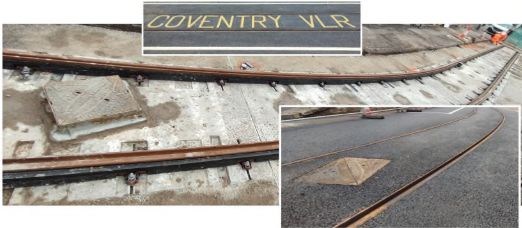
Figure 8: A 36 m (118 ft) pilot installation of the CVLR Track system was completed in 8 single-shift days
