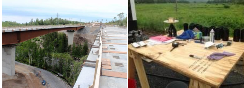
Figure 6: (left) Mackenzie River Twin Bridges – precast concrete decks with UHPC joints (Perry, Krisciunas & Stofko, 2012); and (right) on-site QA/QC equipment.
