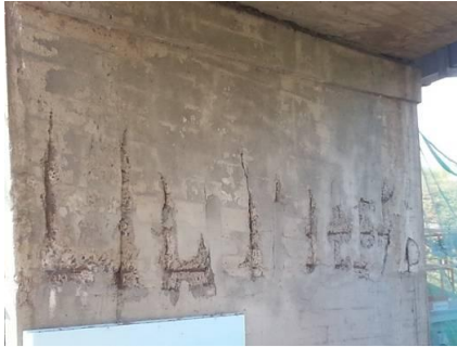
Figure 1. Existing surface before repair
