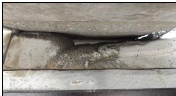
Figure 6. Partially Removed Form Revealing Underfilled Haunch due to Loss of Workability
