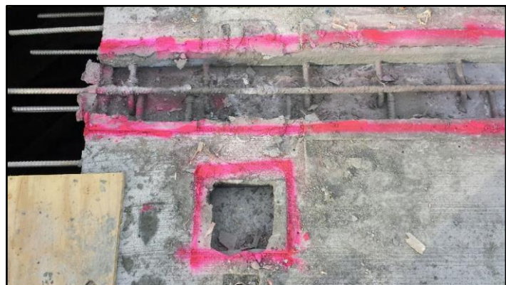
Figure 7. Underfilled UHPC Panel Connection and Shear Pocket Due to Leaking Forms
