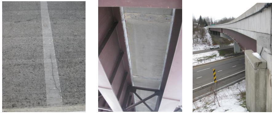
Figure 15. Single crack in UHPC connection - No underside leakage – Bridge structure
