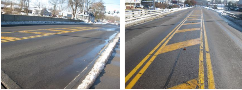
Figure 7. Deck surface with centerline longitudinal cold joint
