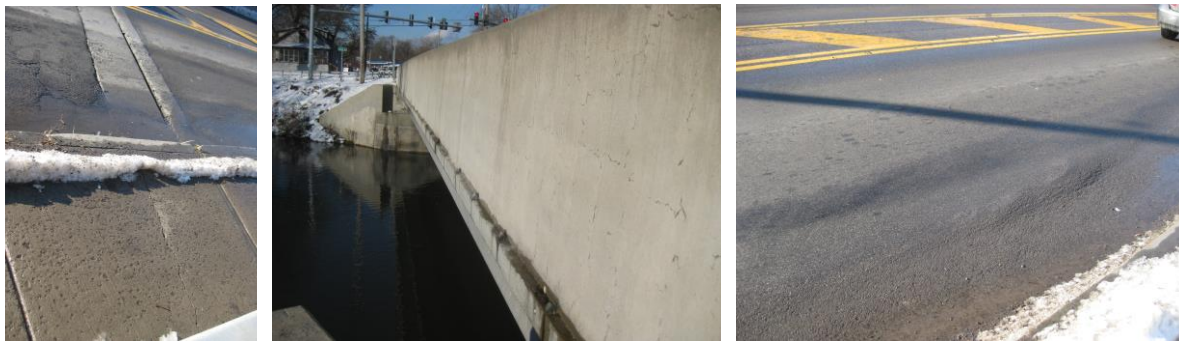
Figure 8. Excess sidewalk scaling, expansion joint failure, ASR cracking and asphalt rutting
