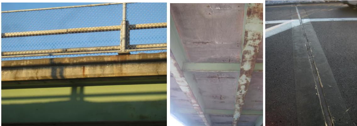
Figure 13. Deterioration of existing bridge deck and expansion joint at abutment
