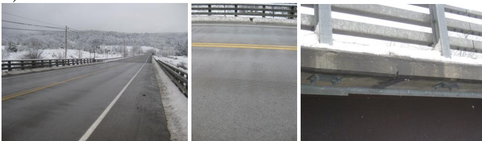
Figure 9. Deck Surface – No reflective cracking on top of panel-to-panel connection; wear & tear of grooving
