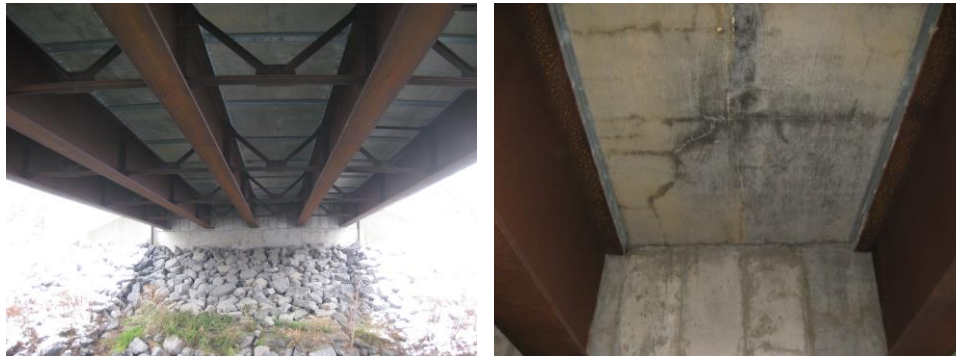
Figure 10. Underside Inspection - No leakage through UHPC connection; Full depth crack in precast panel
