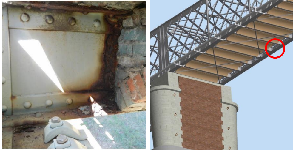
Figure 2: Corrosion pathologies of the bridge
