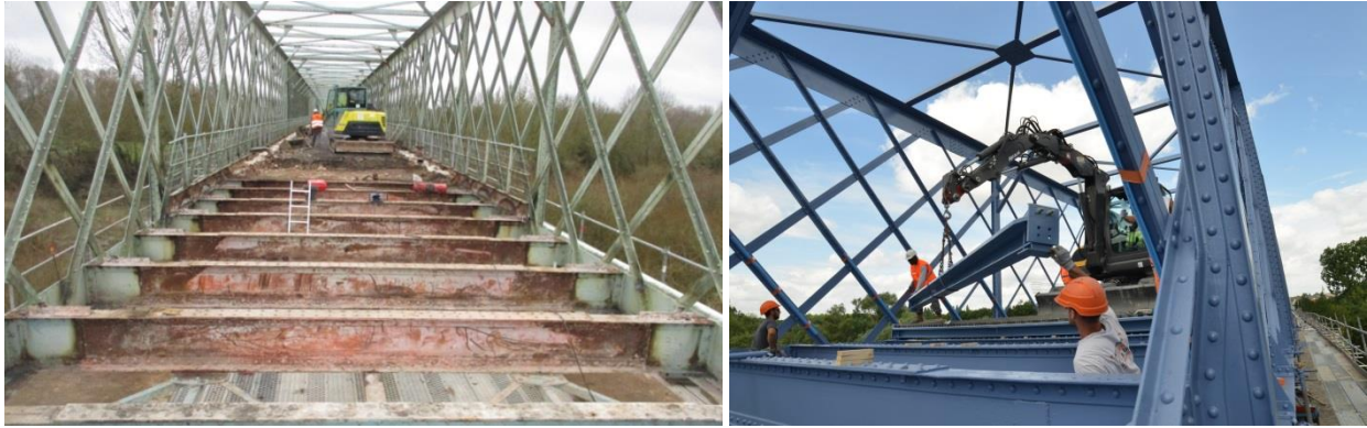
Figure 6: Pictures of brick masonry arches demolition and of new girders installation after repainting.
