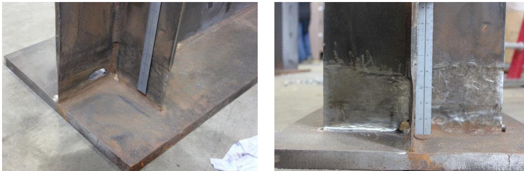
Figure 2: Simulated corrosion damage
