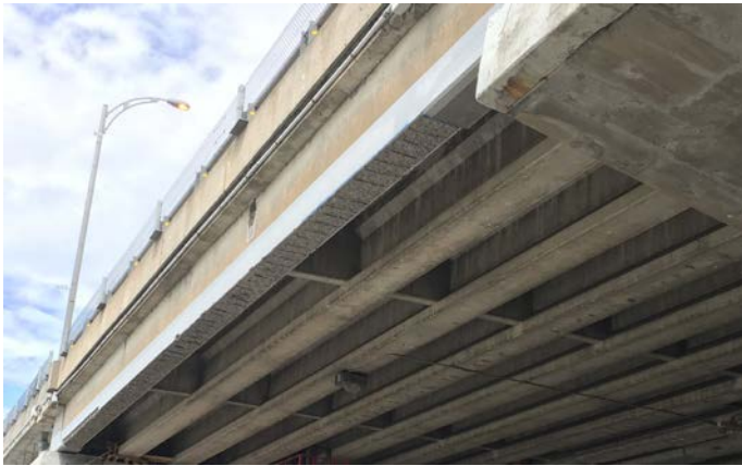
Figure 1 - Bottom view of the viaduct (bottom flange concrete has been removed)
