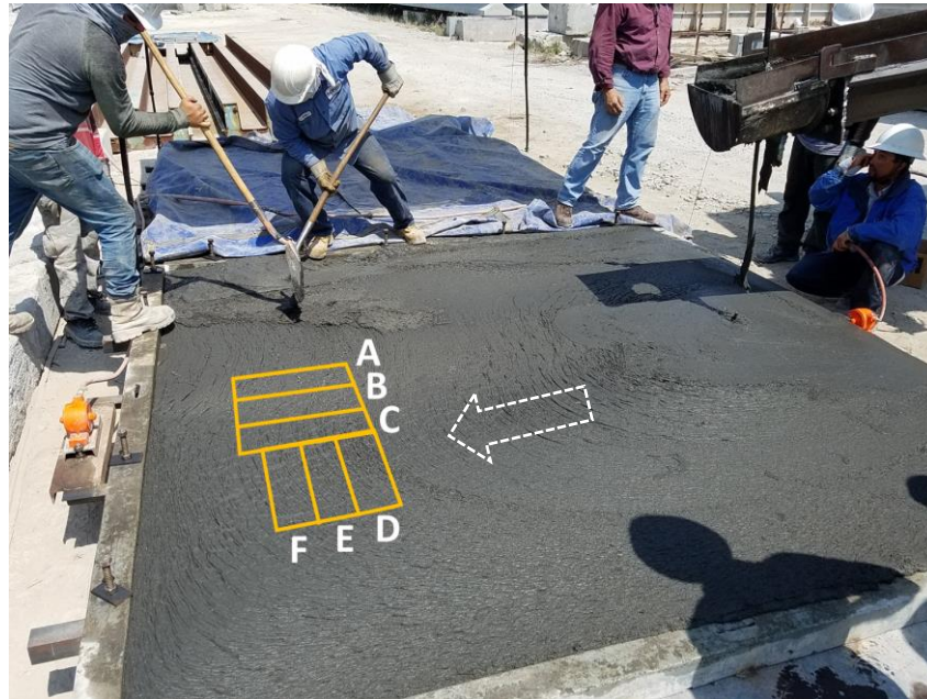
Figure 2. Filling of panel forms with UHPC. Approximate locations of cut flexural beam specimens are shown. Arrow indicates direction of UHPC flow.
