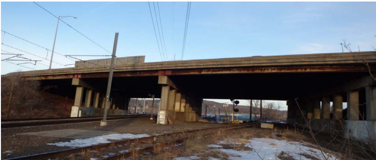
Figure 5. Image of bridge in New Haven, CT scheduled to undergo UHPC repair at beam ends.
