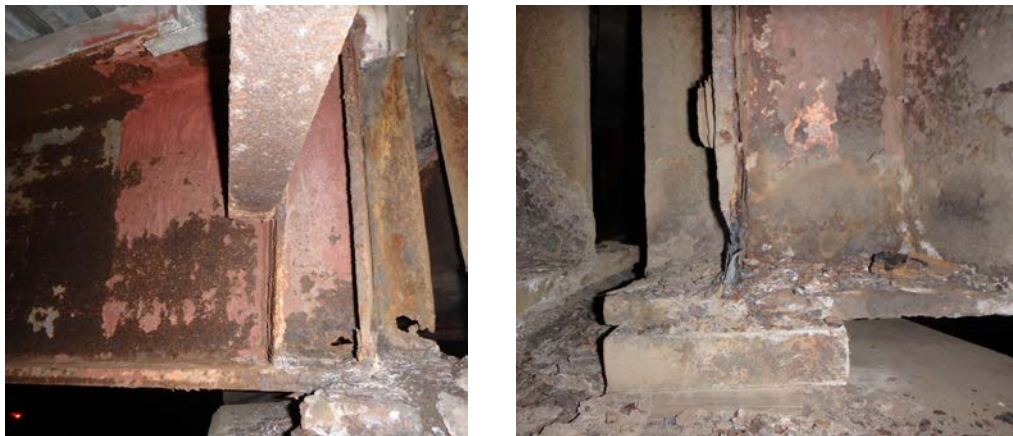
Figure 6. Representative beam end corrosion on the bridge
