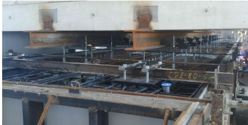
Figure 4. View of the counterweight with the anchoring of lightning polystyrenes and other embedded elements, such as bearings and handling cases.
