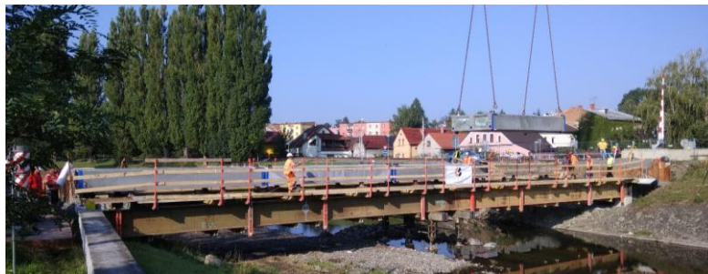
Figure 5. Assembly of the S2 segment (the fourth one in the installation order)
