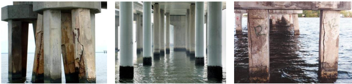
Figure 1. Deterioration typical of precast prestressed concrete piles [Moser et al., 2011, and Griggs, 1987]
